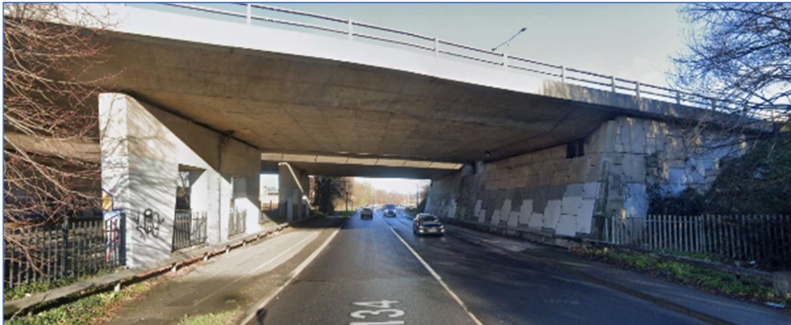
Figure 2.8.8.2 Existing Cross Section at R134 New Nangor Road interface with M50 overbridge
